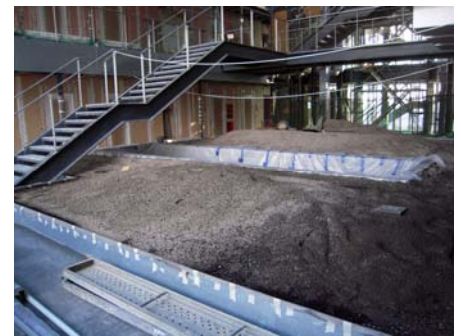
The green roof system build-up "Roof Garden" was applied as a substructure within the planters.
